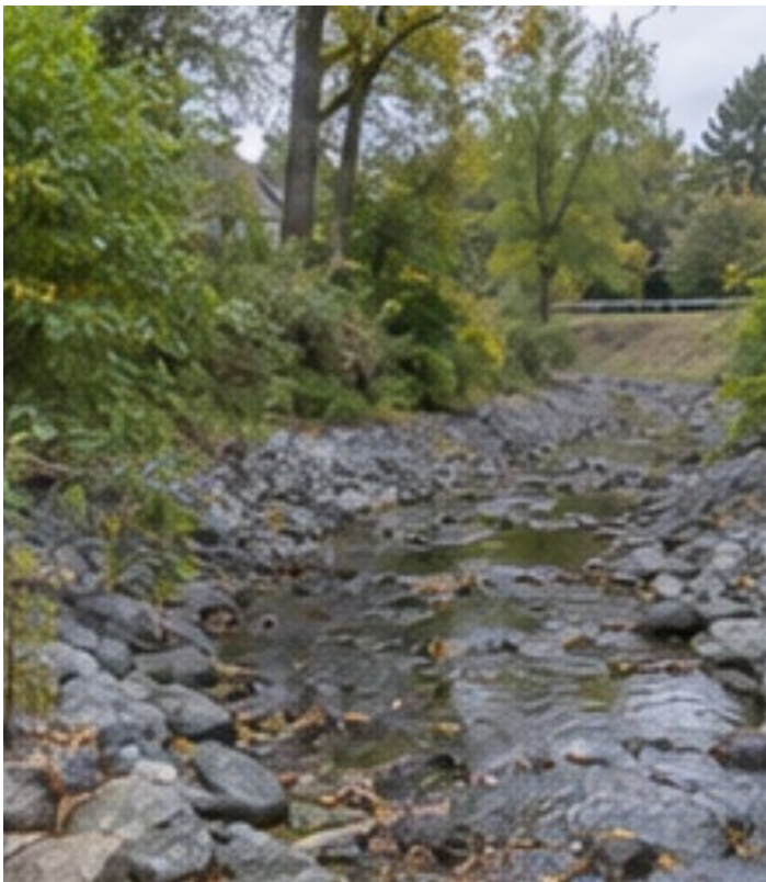
Photo 1: Downstream channel and erosion protection.
