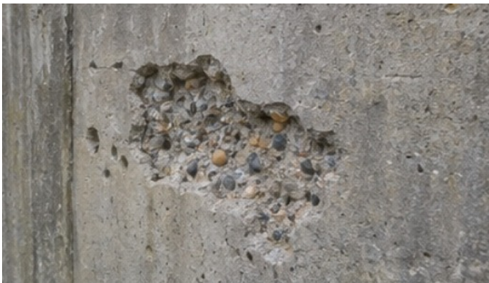
Photo 5: Localized concrete surface deterioration.
