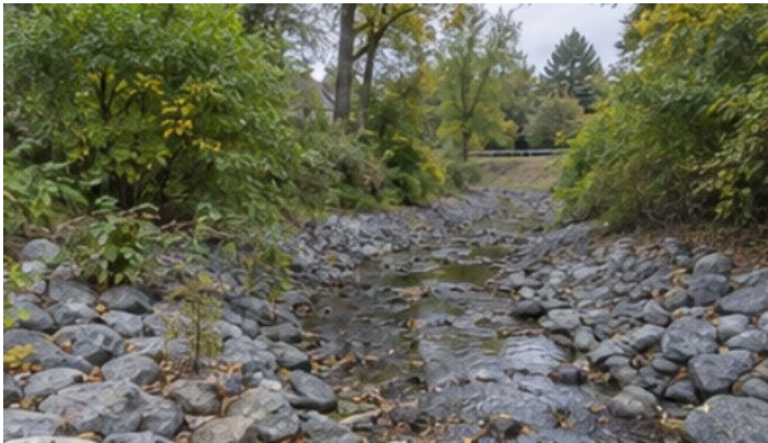
Photo 3: Downstream channel and erosion protection.
