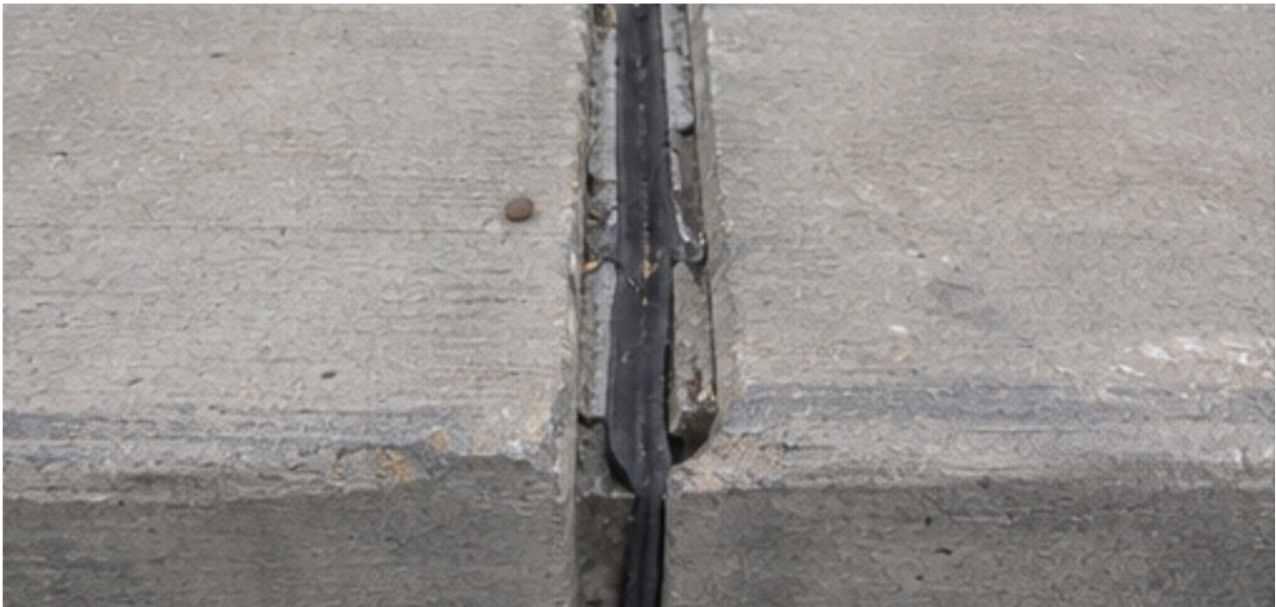
Photo 11: Expansion joint sealant condition.
