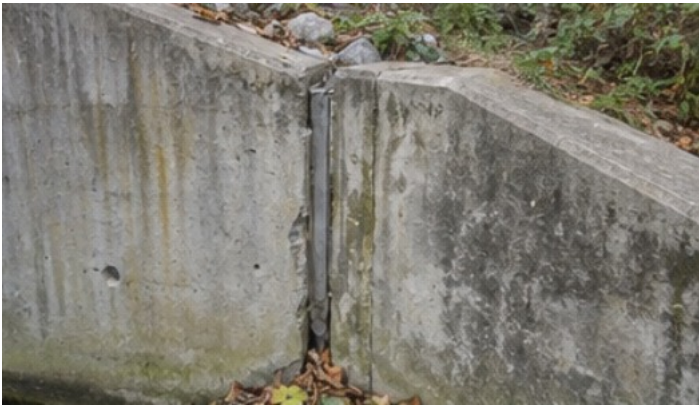
Photo 2: Concrete wingwall joint condition.
