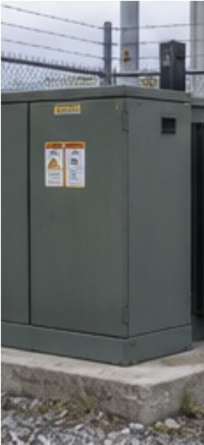
Photo 7: Electrical transformer enclosure.
