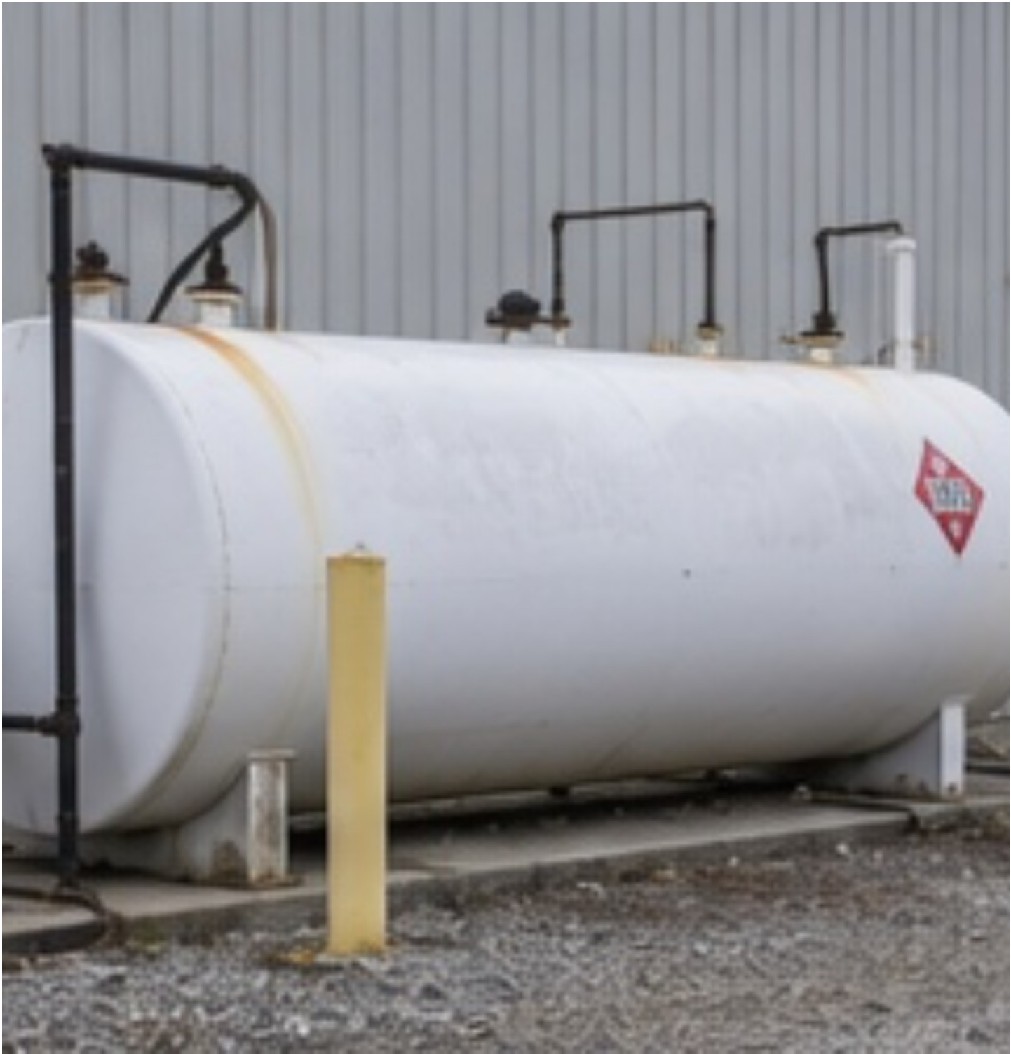
Photo 1: Aboveground fuel tank beside the maintenance building.
