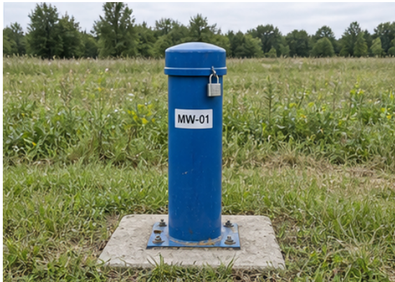
Photo 1: Monitoring well MW-01 and protective casing.
