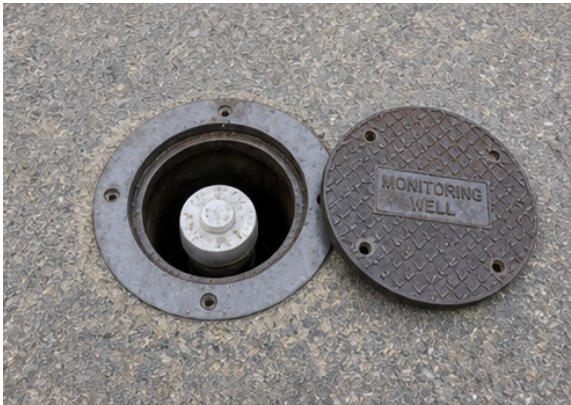
Photo 2: Flush-mount well MW-02 in the service yard.
