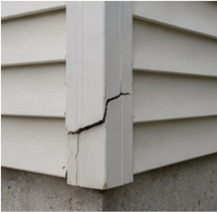
Photo 2: Damaged siding at the building corner.
