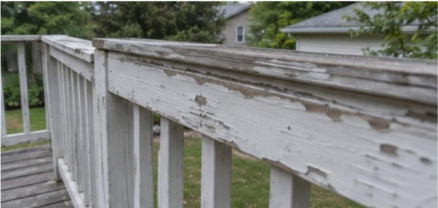
Photo 9: Weathering on the deck railing.
