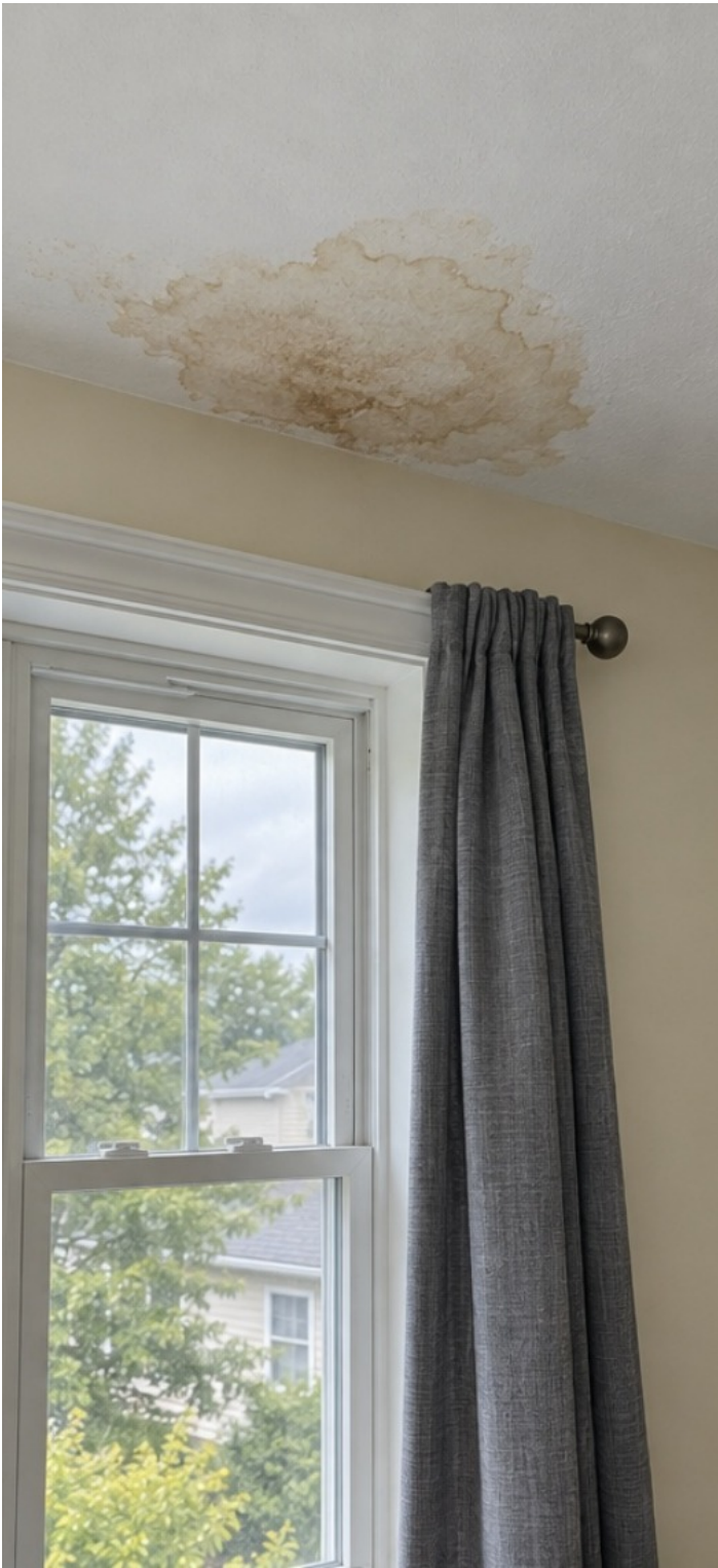
Photo 5: Ceiling staining above the bedroom window.
