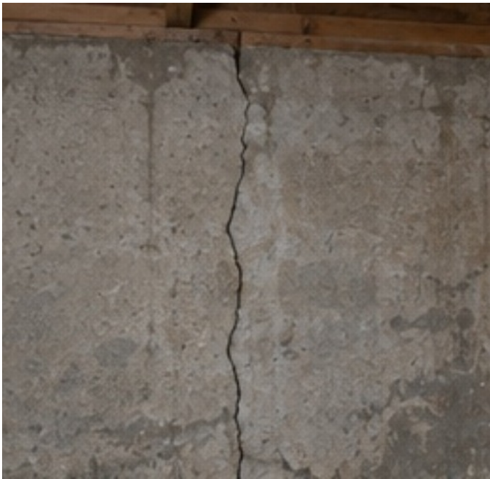
Photo 4: Vertical crack in the basement wall.
