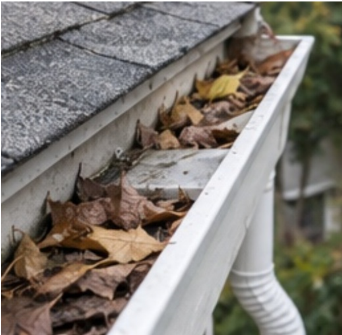
Photo 4: Debris in the gutter near the outlet.
