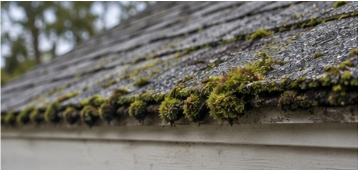
Photo 9: Moss along the shaded roof edge.
