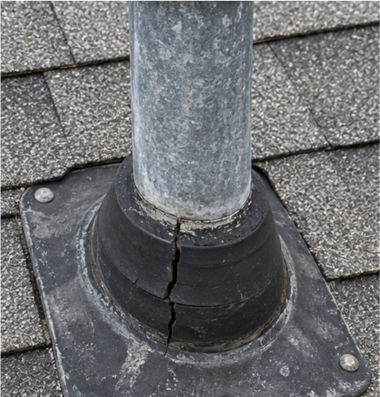
Photo 3: Weathered flashing boot at the roof vent.
