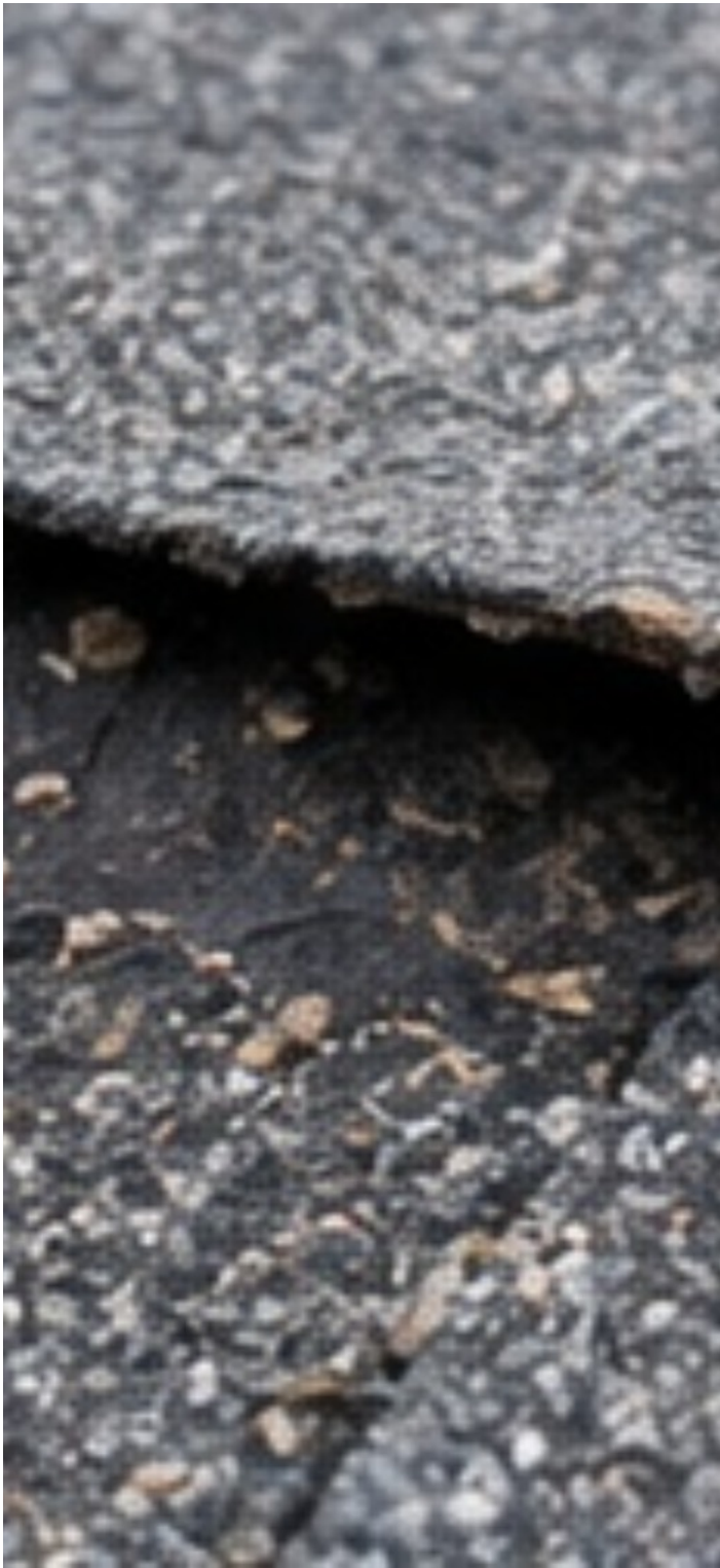
Photo 2: Lifted shingle edge and granule loss.
