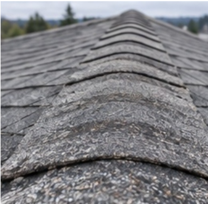
Photo 6: Condition of the ridge shingles.
